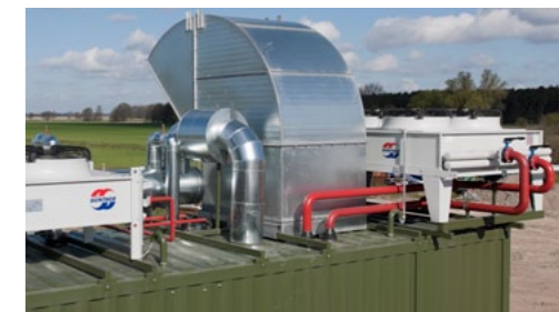
Unit on the left: The Güntner GFH drycooler serves as oil-mixture cooler; unit on the right: The Güntner GFH drycooler serves as emergency cooler that can be used e. g. during maintenance work on the block heating station.
