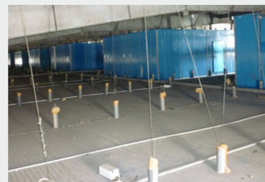
3 One of Vietnam's largest logistics centres is efficiently cooled using NH 3 evaporators and the penthouse concept.
