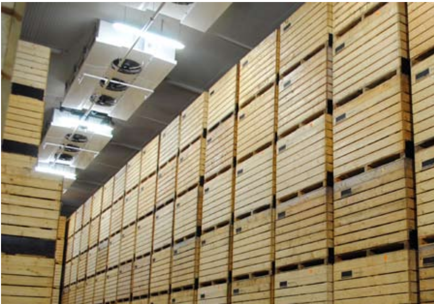
Crates arranged at the Greengrow carrot storage facility with the DGN double-coil air coolers installed in the centre of the room
