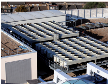
61 Guntner GFH drycoolers ensure low-noise and energy-efficient operation at Westfield London.
