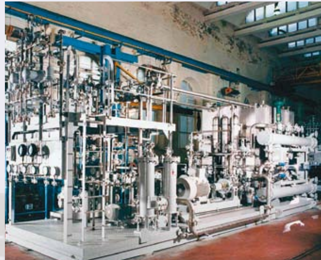
Compressed air cooling
