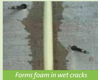
For water bearing cracks
