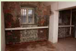
On damp masonry
