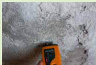
On salt burdened substrates
