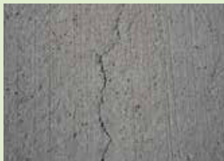
Penetrates into very fine cracks
