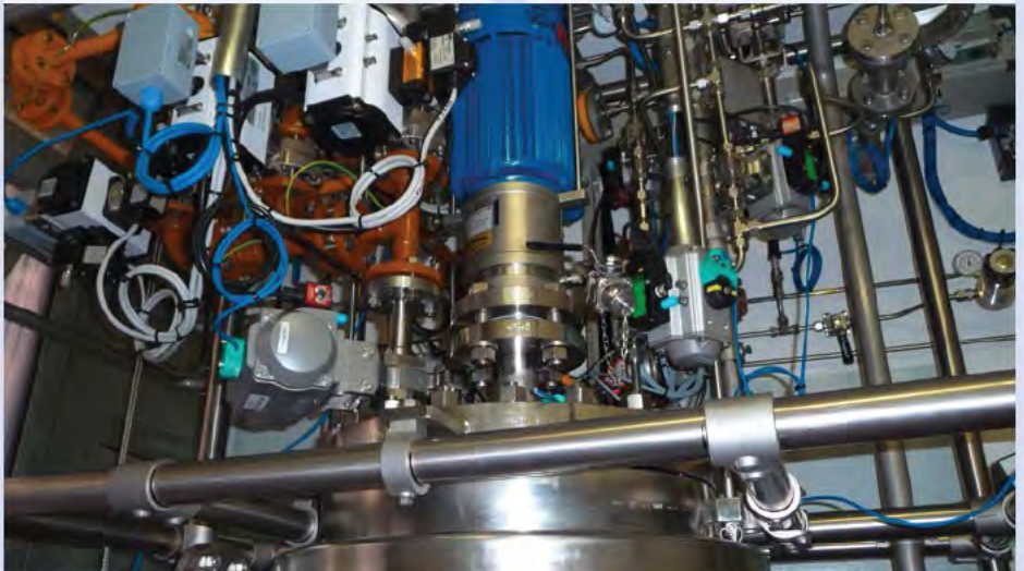
Reactor vessel head with automated valves, Hastelloy, ATEX
