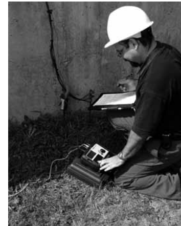
Using ART method with Megger DET3TC to test commercial ground without disconnecting the system
