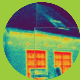
Thermal photograph showing standard cold edge windows - red signifies area of heat loss.
