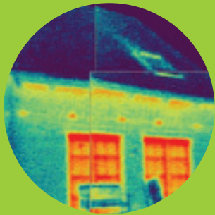
Thermal photograph showing standard cold edge windows - red signifies area of heat loss.
