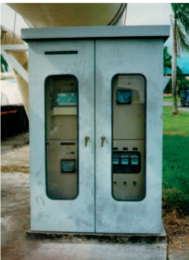
4 Minilog B devices record waste water inflow on a large treatment plant in South East Asia.
