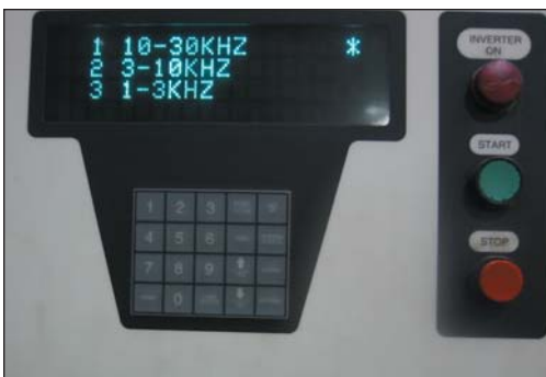
Power source panel frequency display.
