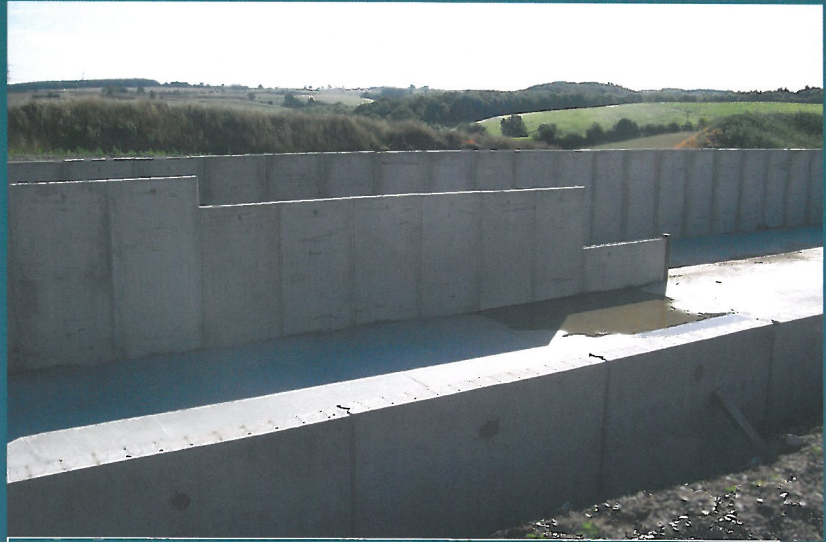
Below ground slurry store incorporating an access ramp for emptying.
