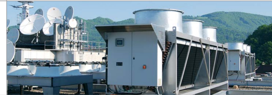
Object (picture left and right): application: data center, coolers: 2 x HTK 1.2/7.2-2S-P2-CU-SLNF, thermal performance: 1600 kW, air inlet: 32°C/38%rH, fluid: water/glycol (30%), fluid temperatur inlet/outlet: 40°C/34°C, controls: HybriMatic single cooler control and HybriMaster control, location: Switzerland, on roof top of a business building in urban environment.
