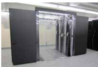
Thermal Curtain Containment
