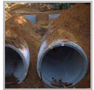
End entry manholes
