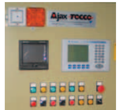
HMI - PLC Control Panel
