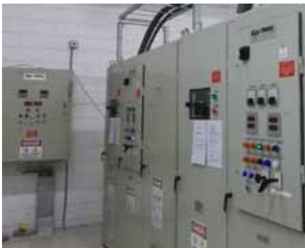
PCU - Power Control Units
