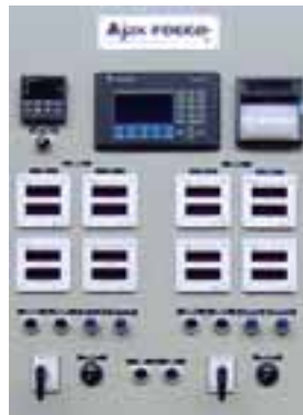
CFC Panel Channel Furnace Control
