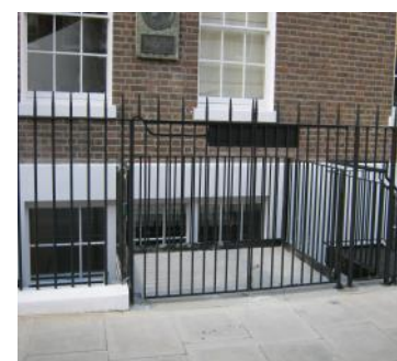
Basement Lightwell Bin Lift in Central London
