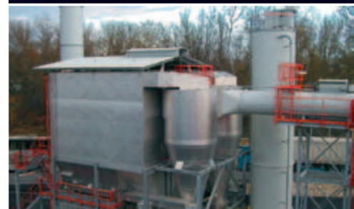
Travelling compressed air – off line – cleaning
