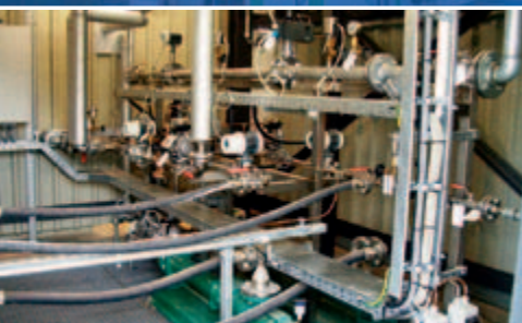
Water/compressed air control station
