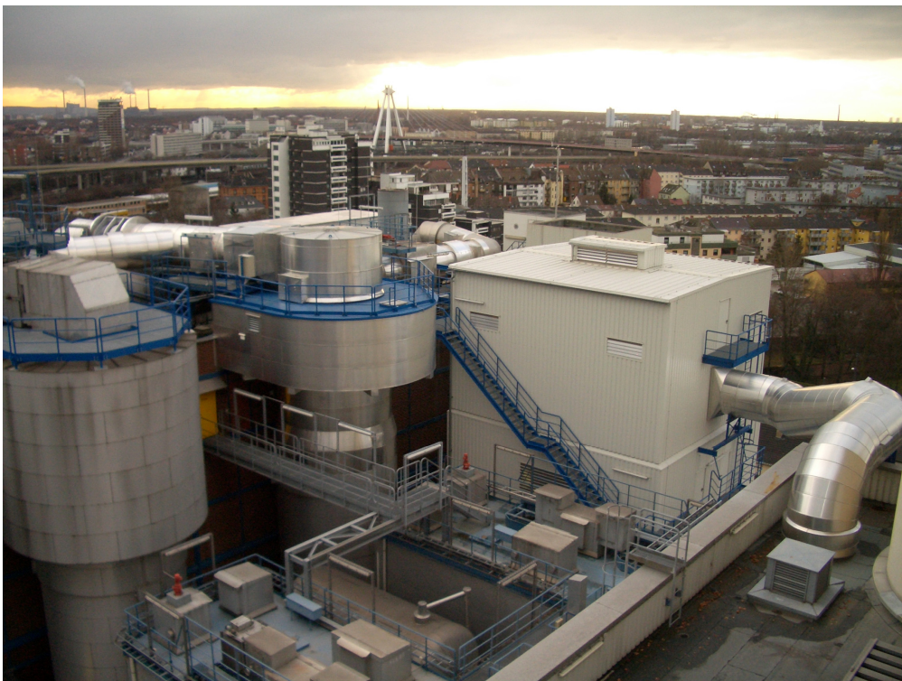
pic. 4: Spray absorber head and filter / reactor building
