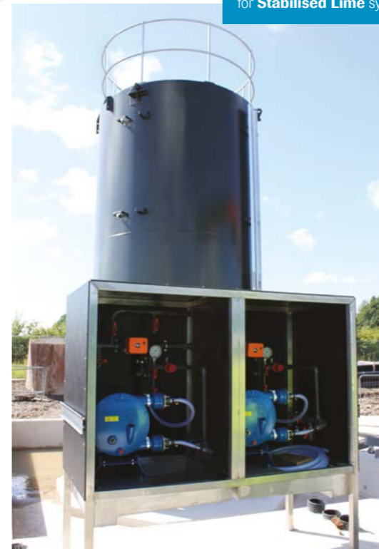
Installation of chemical tank and dosing pumps for Stabilised Lime system
