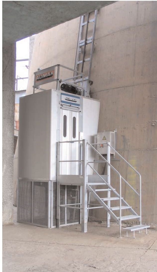
The Alimak lift is used for emissions monitoring and general inspection of the chimney stack at the coal-fired power plant outside of Bobov dol, Bulgaria.
