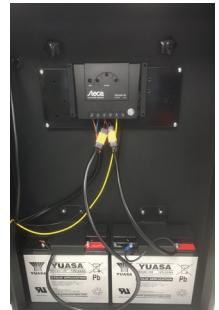
2 batteries and Solar Charge Controller
