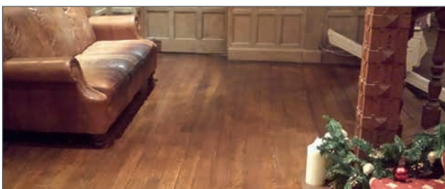
▲ Deep clean and re-polish of this tired wooden floor. The results were amazing.
