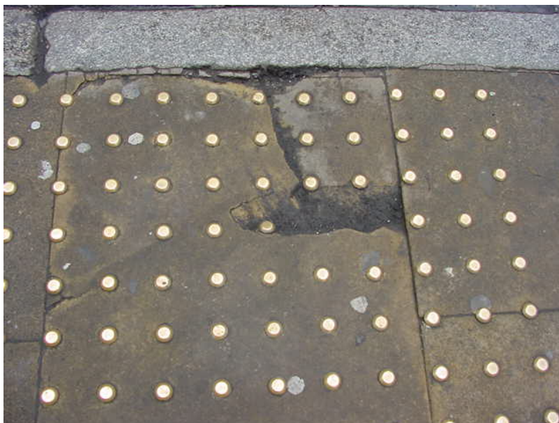
Figure 4.10 Detail of the pedestrian crossing at the junction of St. Wurberg Street and Eastgate Street. Installation of the studs appears to have weakened paving, causing a potential trip hazard.
