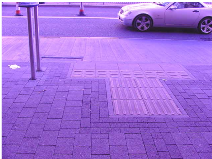
Figure 4.5 Bus stop on Arundel Gate. Buff lozenge tactiles have been incorrectly installed to indicate on street bus stop, directional guidance path tactiles have been installed leading to the bus stop.
