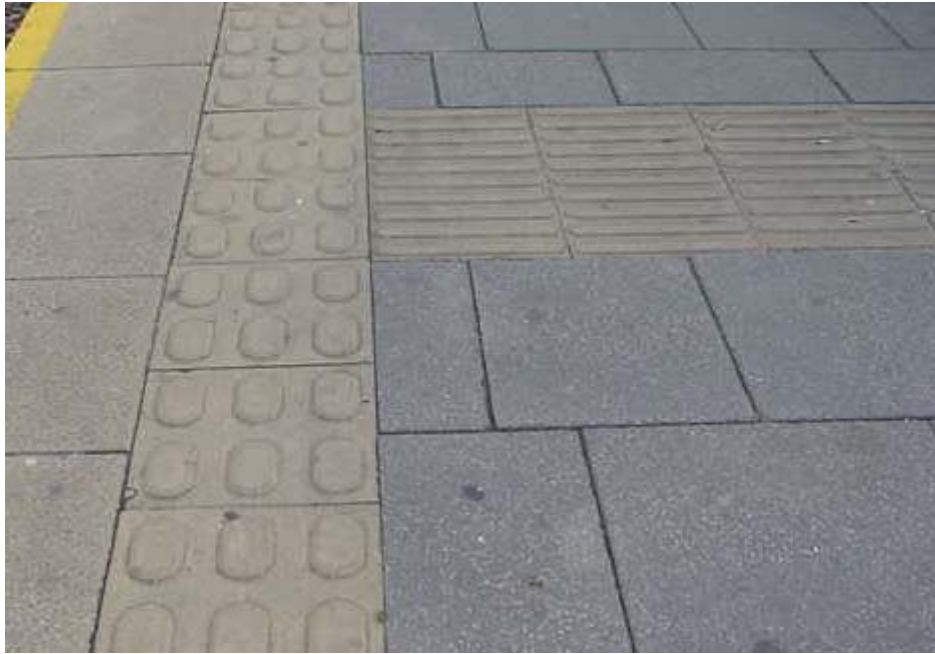
Figure 2.8 Example of correctly installed lozenge tactile paving at a tram stop.
