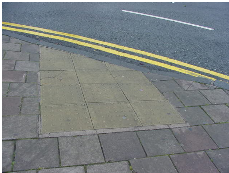
Figure 4.7 Junction of Newgate Street and Pepper Street. Example of buff concrete blister tactiles installed at an uncontrolled pedestrian crossing point.
