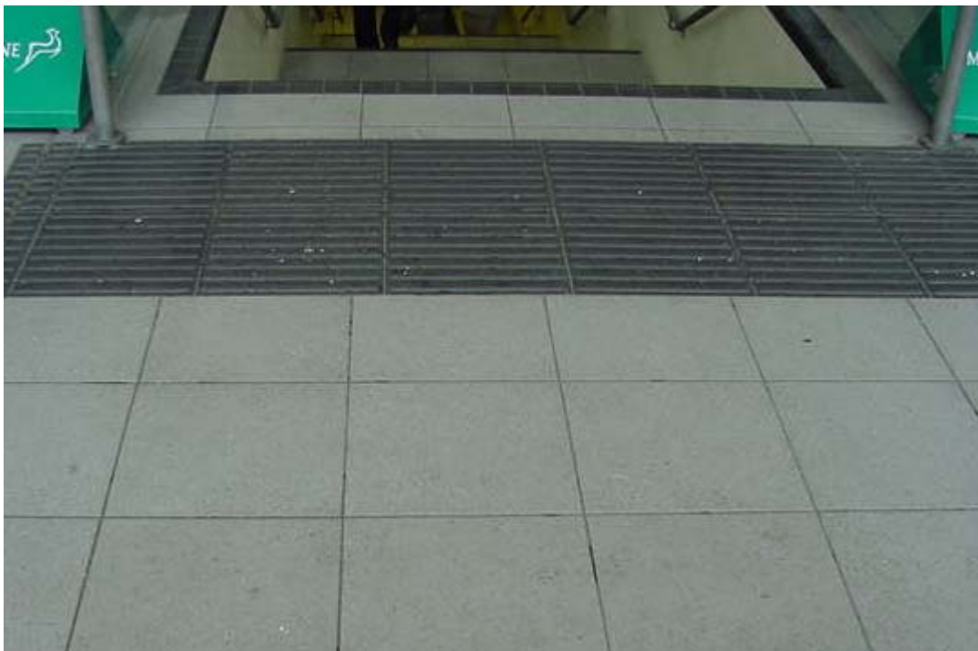
Figure 2.10 Picture of correctly installed corduroy tactile with good colour contrast with the surrounding floor.
