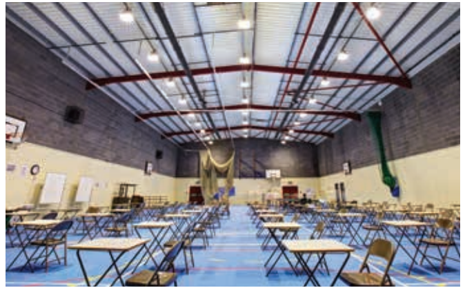
Abbey Gate College, Cheshire, UK White high bay lighting installation
