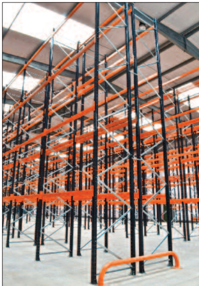
We have a wide range of pallet racking solutions to meet your operational needs, whatever your warehouse size.
