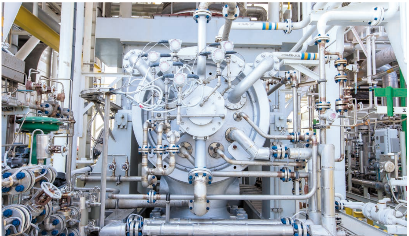
Multi-channel monitoring of compressors and piping
