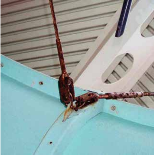
Severe corrosion / catastrophic degradation after less than two years in service
