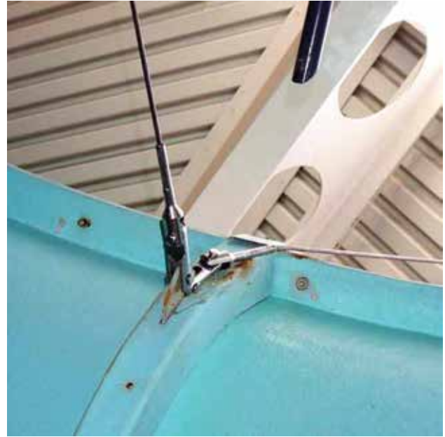
Completely corrosion free after more than eight years in service
