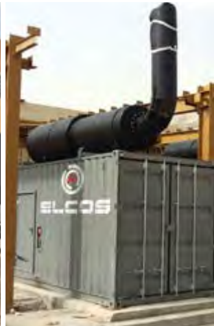
FAR EAST POWER PLANT 3 X GENSETS IN CONTAINER 2
