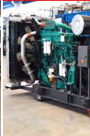
800 KVA BF WITH DUAL BATTERY SYSTEM
