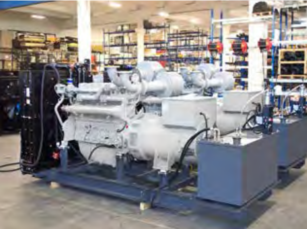
800 KVA WITH DOUBLE WALL TANKS 1000 LTS
