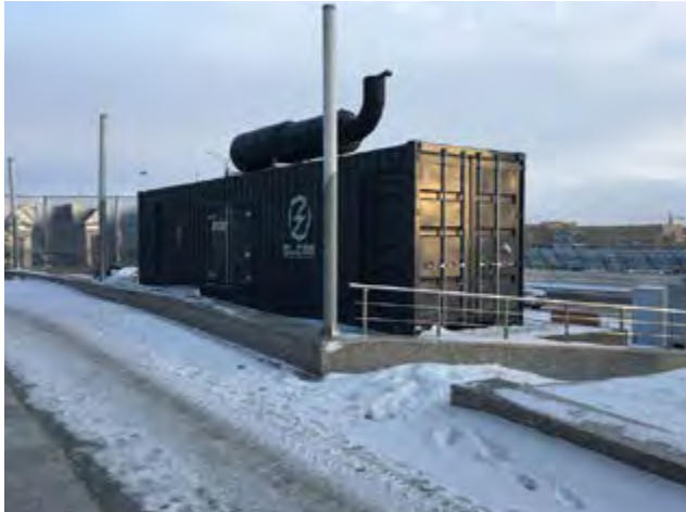
KAZAKHSTAN GENSET IN CONTAINER 40'1880/1700 kVA
