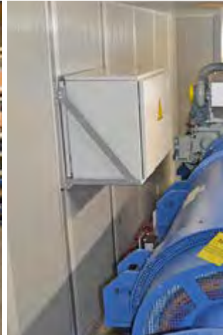
GS WITH NO BREAK DOWN IN CONTAINER
