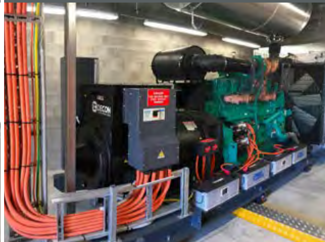
AUSTRALIA 2 X BASE FRAME 825/750 kVA
