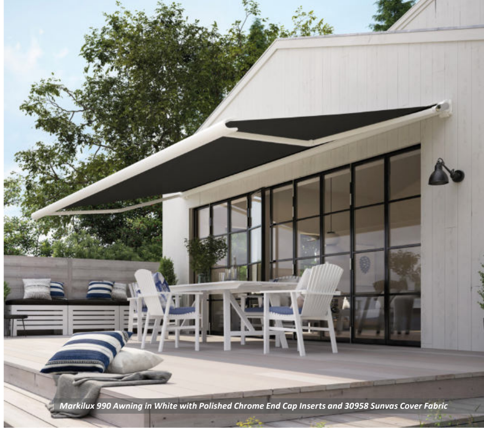
Installation of five Markilux 990 Awnings in White with Pattern 32860 Sunsilks Cover Fabric
