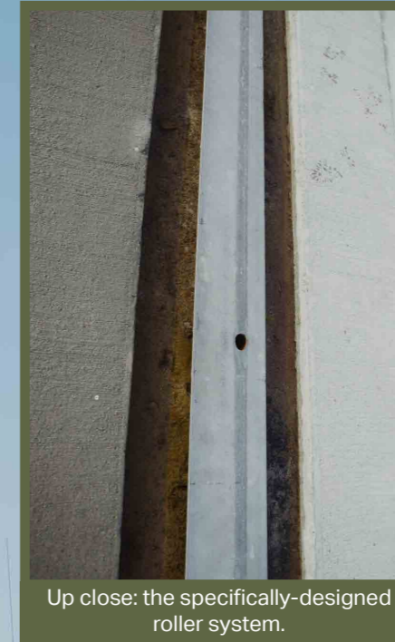
The building will pull back along these rails to reveal the asset.
