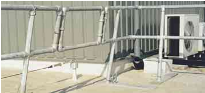
Safe access points can be formed within the system.
