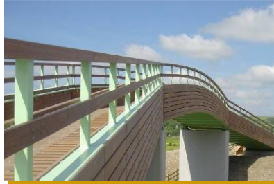
Steel beams clad with hardwood fascia and painted steel parapets with hardwood rails
