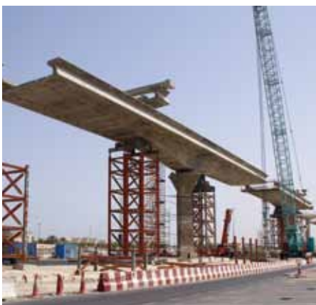
Work on projects like the Dubai Metro in the Middle East have helped RMD Kwikform to expand overseas
