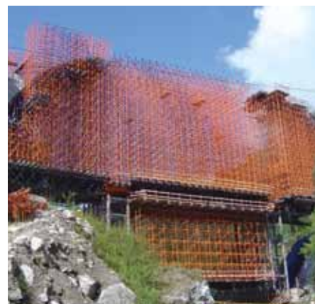
Overcoming engineering challenges to construction the Bridge over the River Homen in Brada, Portugal
