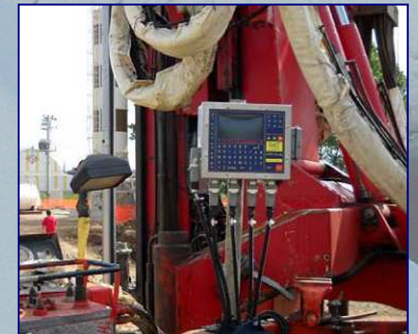
DAT instruments JET 4000 AME / J - MD data logger on drill rig at construction site
