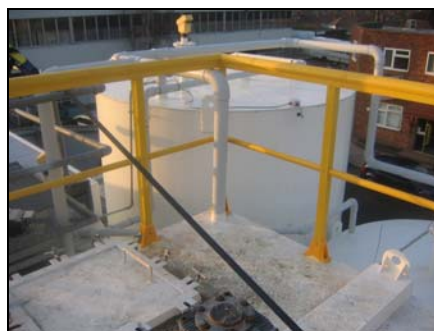
Yellow handrail system
