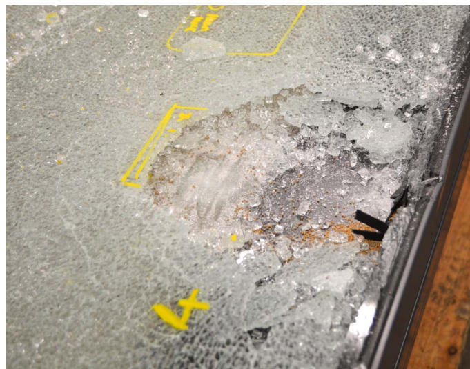
Example where toughened outer pane has shattered under attack, but laminated inner remains intact (note frame damage where hand tools have been levered).
