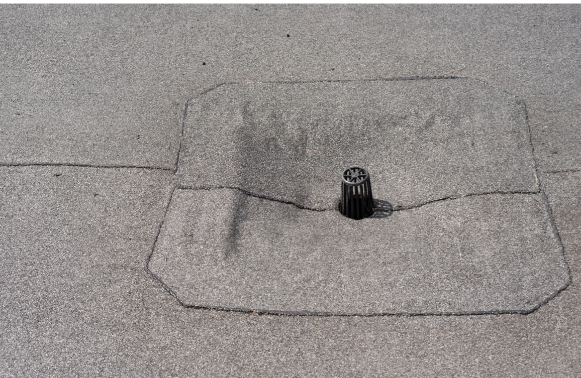
Drainage system installed in felted flat roof.
